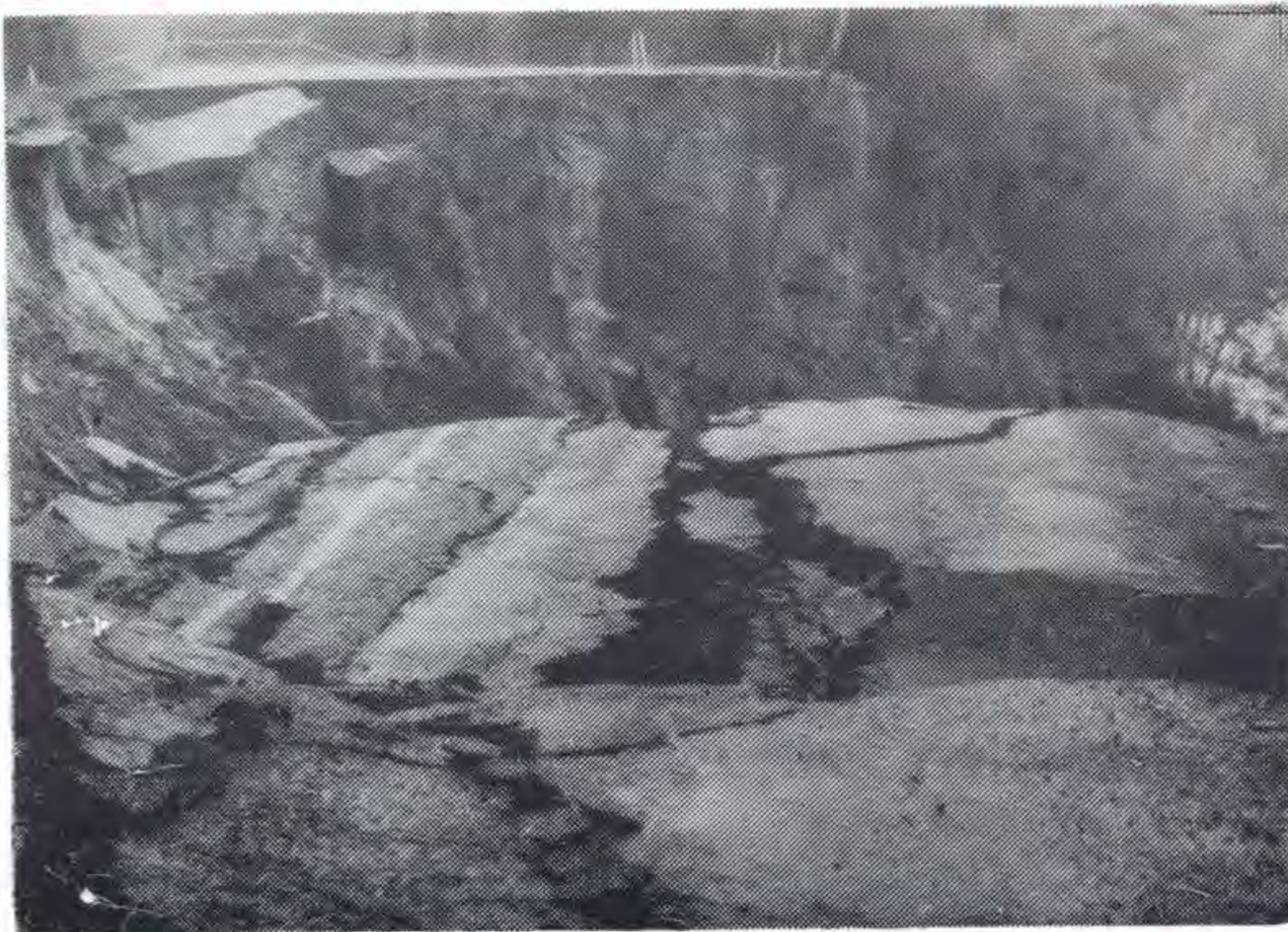
Above: Looking more like a scene from the movie 'Earthquake' this striking picture of the washed away road was taken in the rain by CONTACT photographer Terry Smith.
