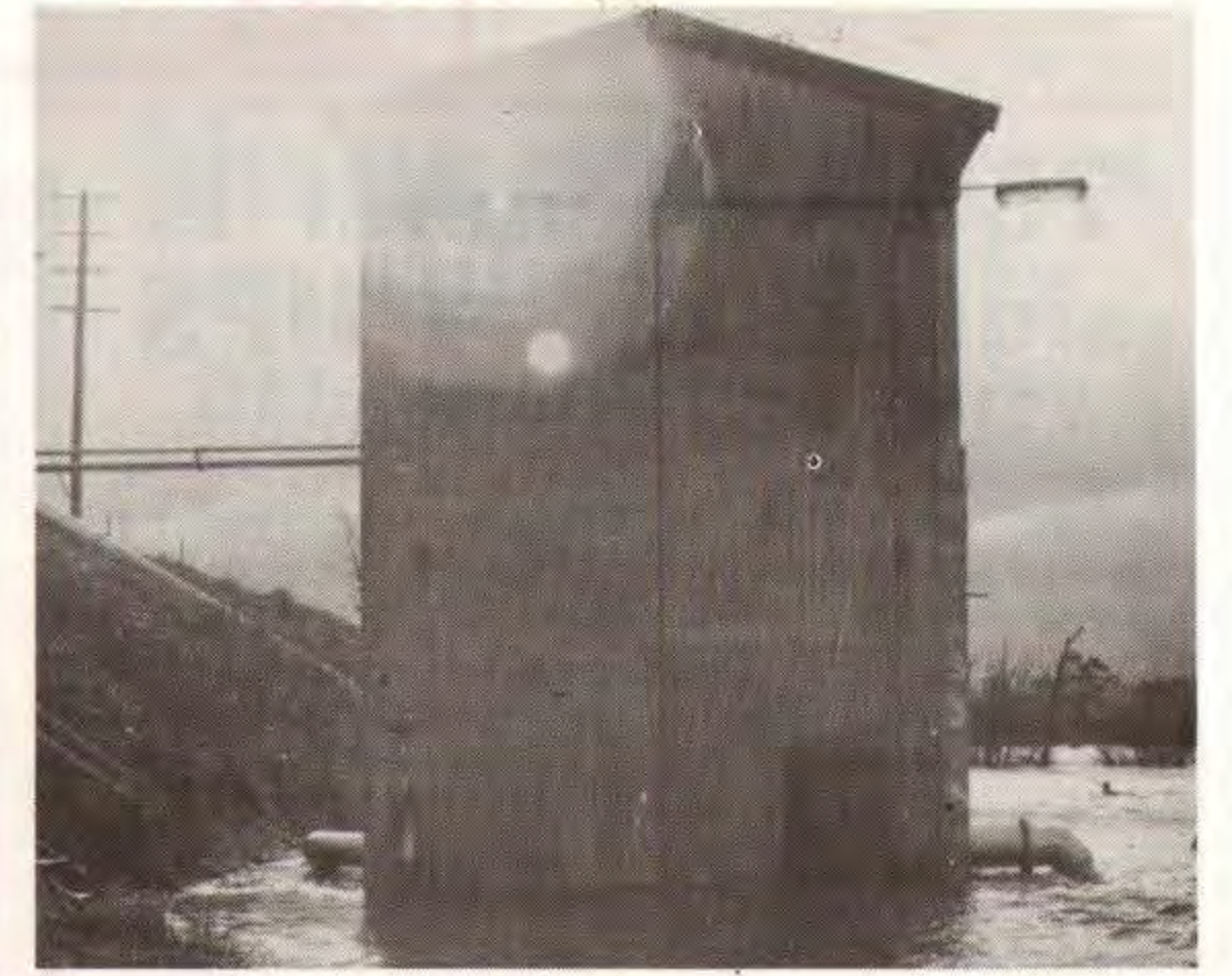
Below: This pump station on the eastern side of the Eastern Levee Road at Yallourn had water from the flooded Morwell River rushing through it.
