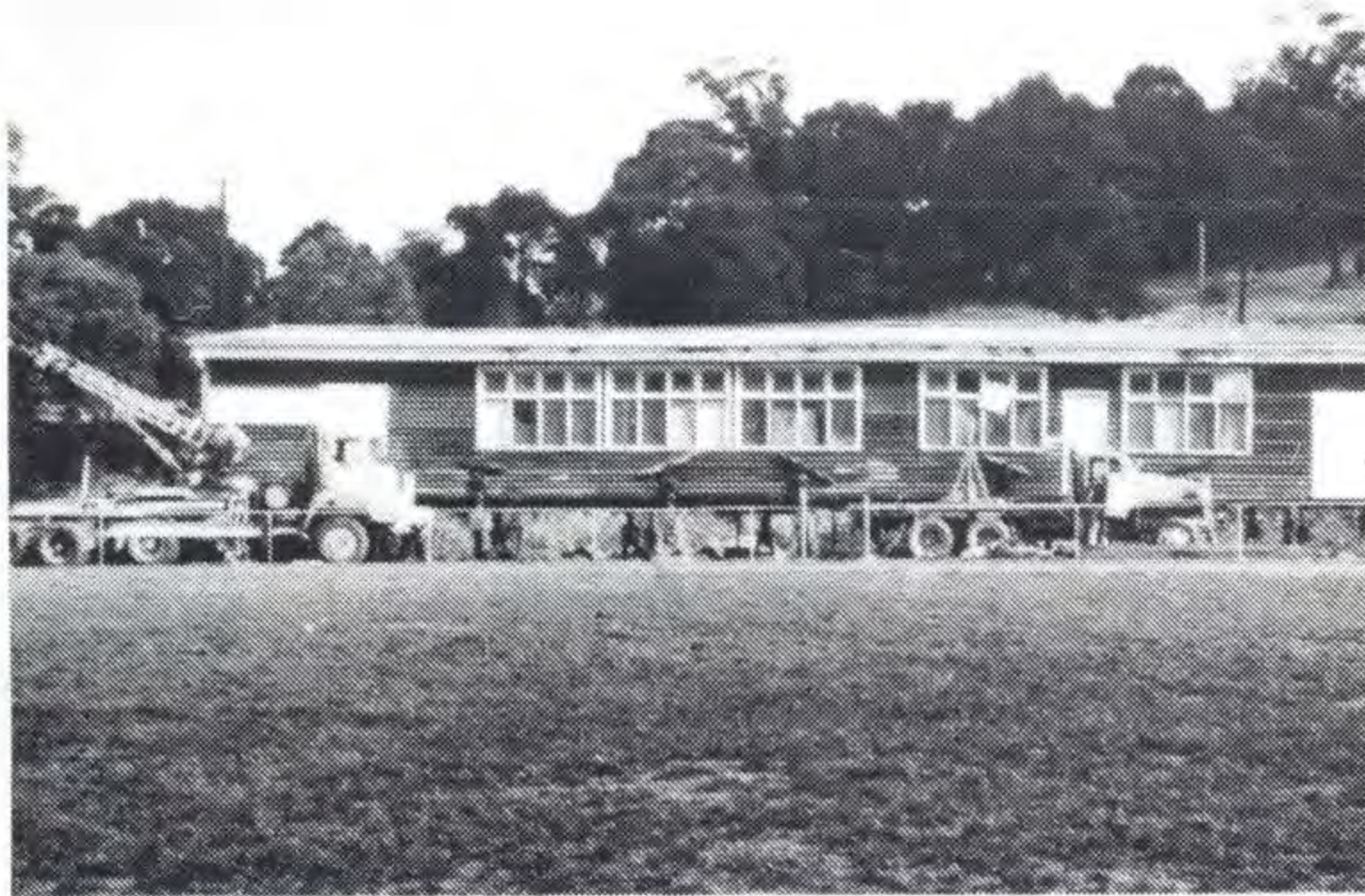
The re-sited pavilion is pictured (right) being placed in position by contractors, Fowlers of Trafalgar. The newly constructed oval is pictured in the foreground.
