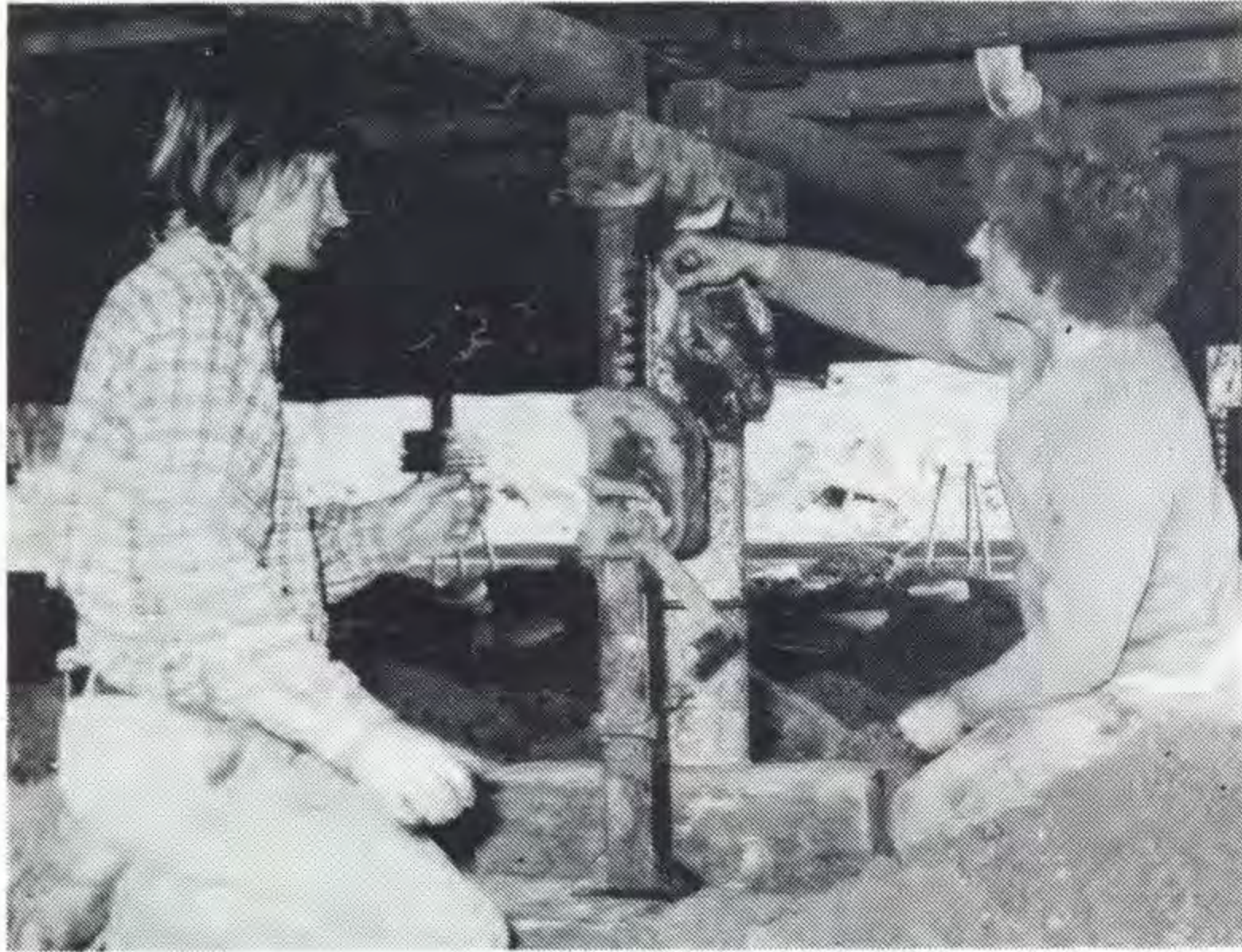
Two workmen make adjustments to one of the many jacks which supported the Hernes Oak pavilion before it was lowered on to foundations early this month.
