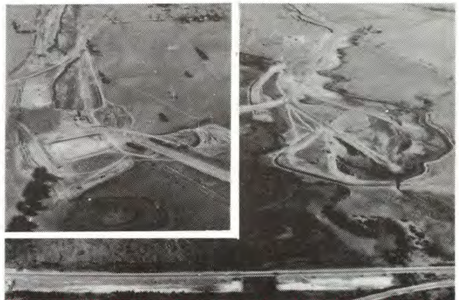
Two aerial shots (above) of the diversion give you a better idea of the extent of the works. The Insert shot, was taken from the south, while the larger picture was taken from the North, with the Princes Highway in the foreground.
