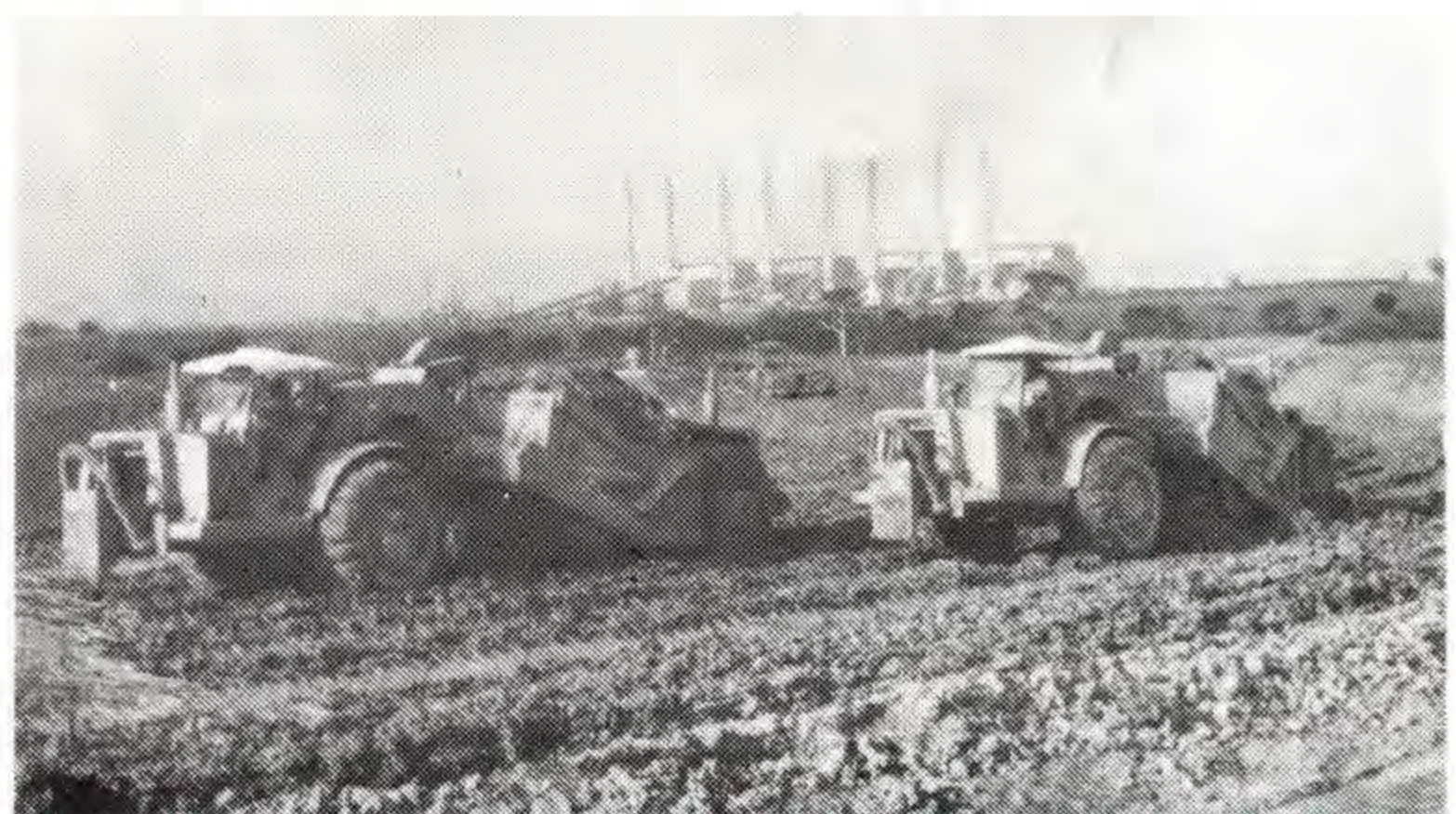
Two large scrapers operated by sub-contractor J. Jeffrey and Sons of Morwell are pictured busy at work on the Eel Hole Creek diversion works.
